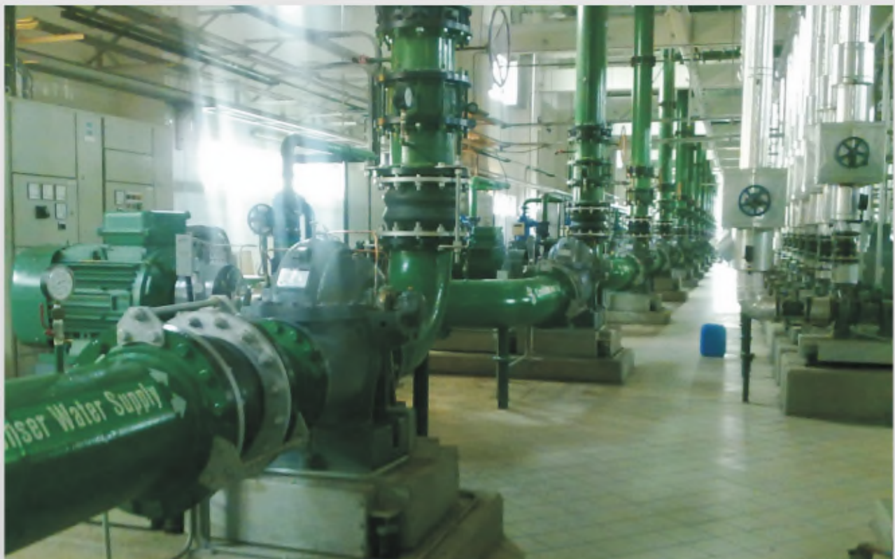
Kuwait University plant room, Kuwait
